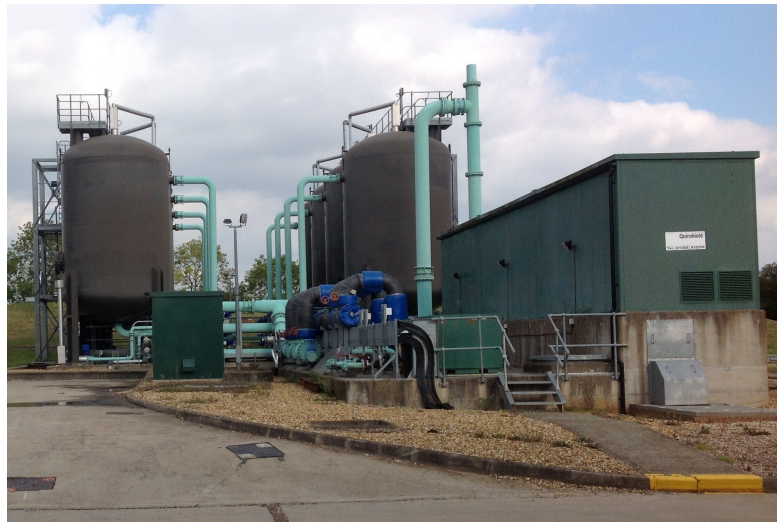
Activated carbon filters at Campion Hills
